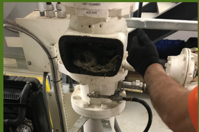
Pump cleaning to remove build up from wipes and paper towels
