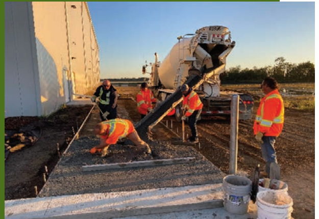
Transportation: MLC – east sidewalk install for COVID-19 building exit plan and proper backfill and drainage along east side of building
