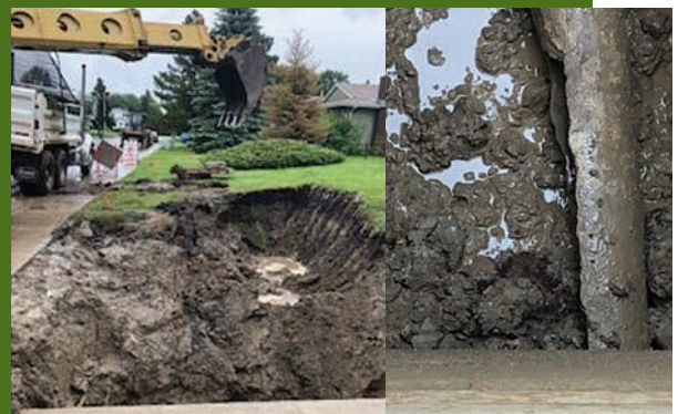
Large waterline beam break on 99A Ave where the main line was within the property line of the homeowner.
